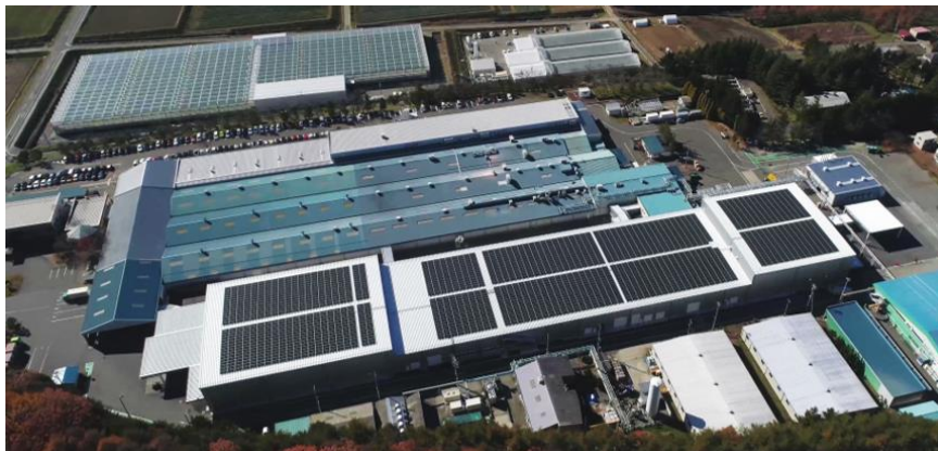
Solar panels installed at Fujimi Plant
