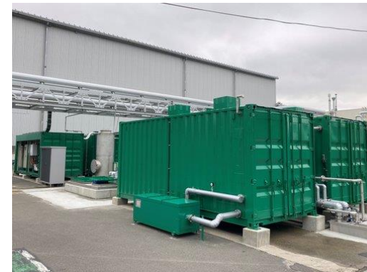
Biomass power generation facility at Fujimi Plant
