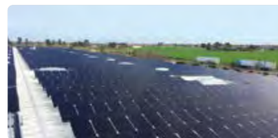
Solar panels installed at Kagome Inc. (United States)
