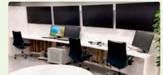
Centralized control room
