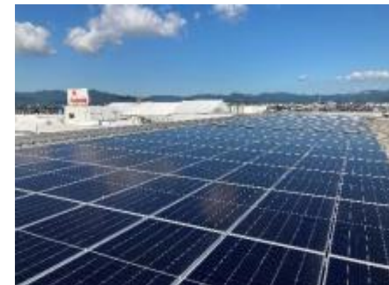
The Kozakai Plant where solar panels are installed
